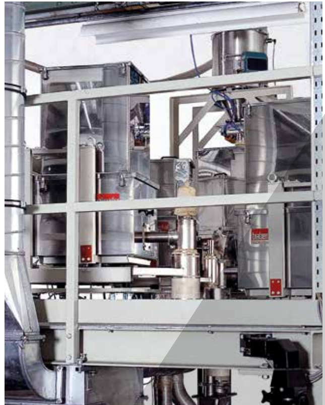
Gravimetric feeders in operation
